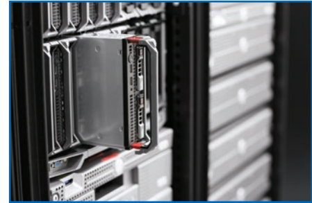
High-density loads like blade servers and PoE switches can create hot spots that traditional perimeter cooling systems have trouble addressing.
