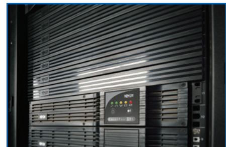
Simple steps like installing blanking panels in unused rack spaces can help prevent warm air from recirculating and improve cooling efficiency.
